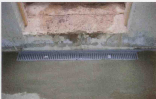
Floor grate at bulkhead door ties into system.
